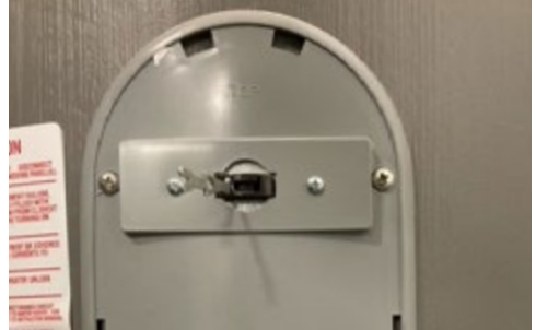
The lower element disconnect in the ON position. (To the left)
